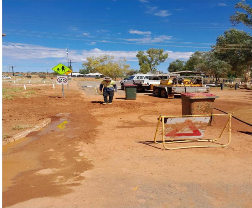
FIGURE 3. Water pipe burst.
