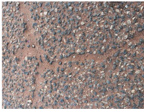
Road surface is thin. This is earth that can be seen through the road
