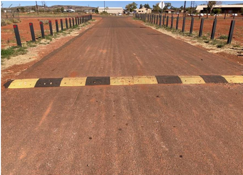
Road Humps throughout the Kintore Area require YELLOW fluorescent paint as part of WHS compliance. This is a rare footage of a road-hump whose colour has not faded.
