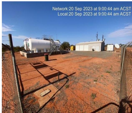
Finke (Aputula) Power Station Compound
