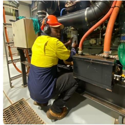
Finke (Aputula) ESO (Relief), servicing generator.
