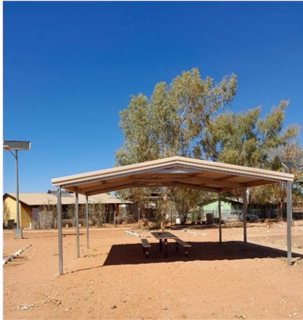
Middle park no concrete floor.
