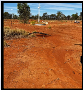
Damaged pipe at Warren Creek Outstation
