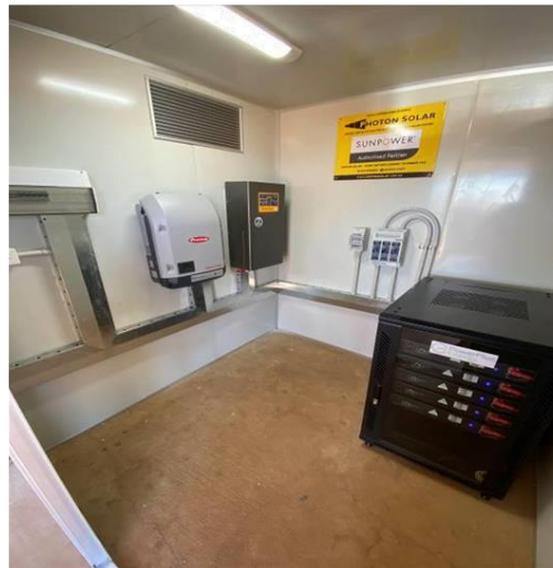
Upgrade to Solar at Amunturrngu Springs
