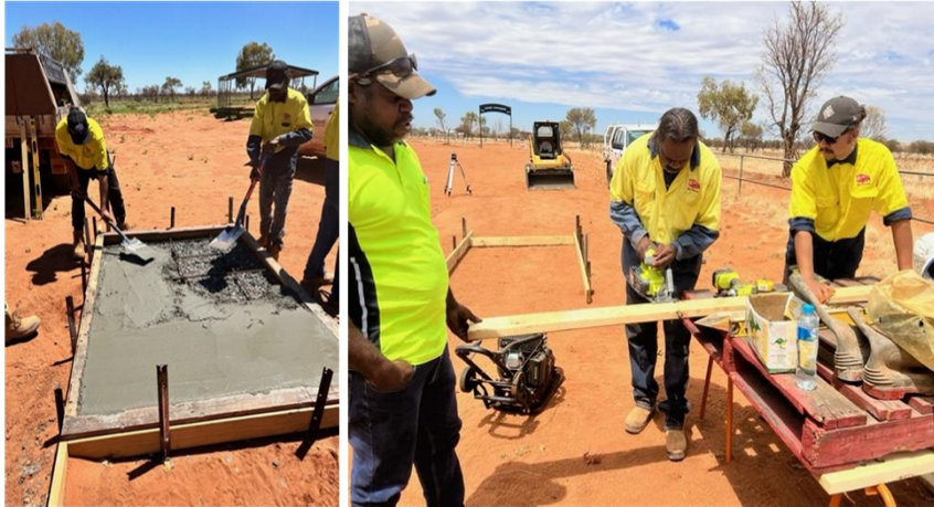
Fig 1 and 2 civil team working on the base for the shed at the cemetery
