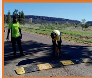
Derek Hayes and Henry Oliver from Amoonguna repairing speed hump and signs
