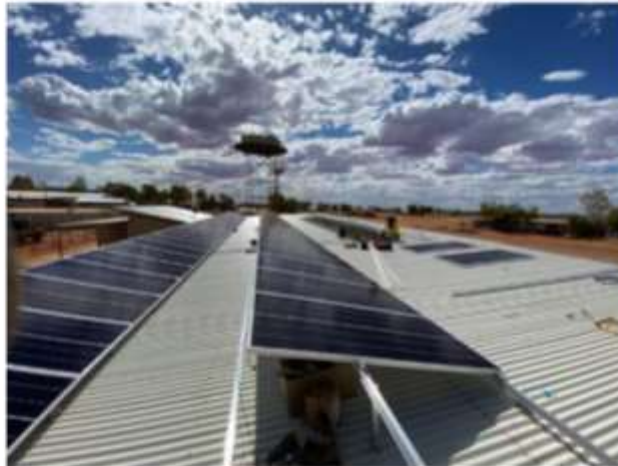
Solar panels on SCD office, Papunya
