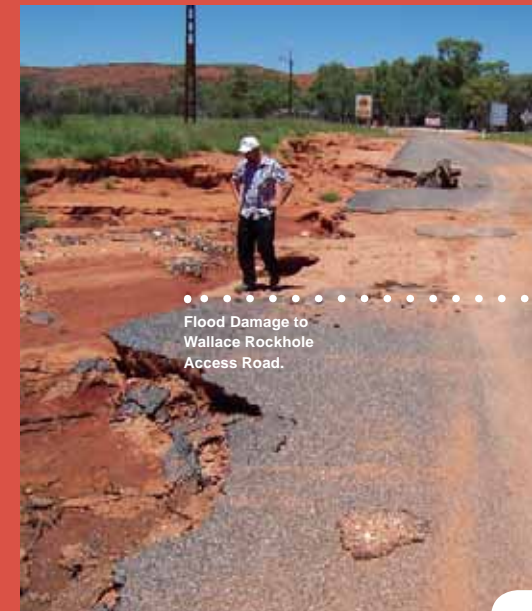
Flooded Highway on the way to Aputula, February 2010.
